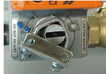
High Fire Position
