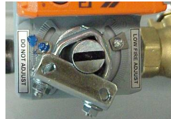
High Fire Position
